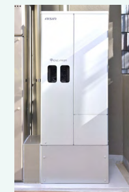
ENE-FARM system installed in a dwelling unit
